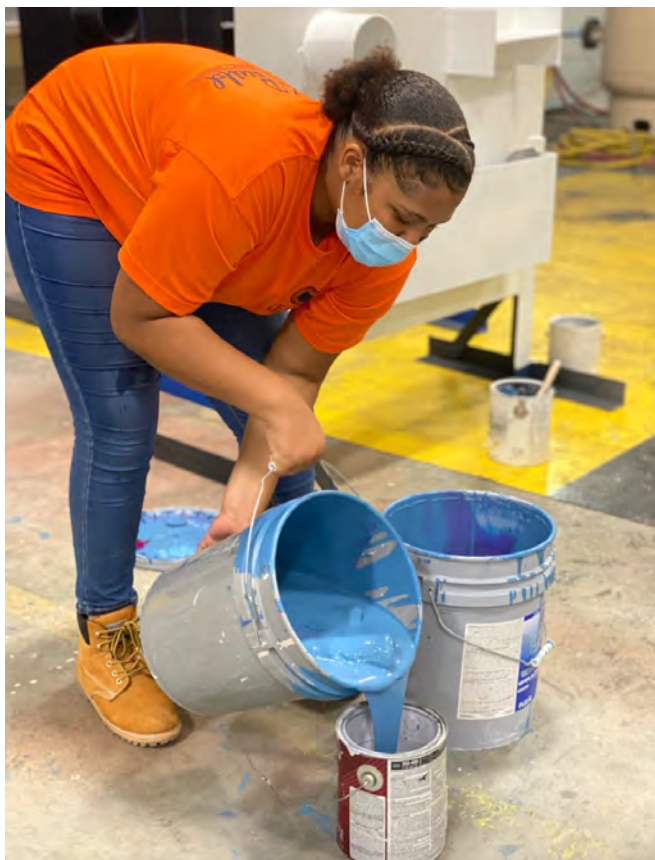
Ashae pouring the paint into the bucket getting ready to paint the wall.
