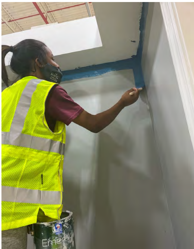
Simone is painting the corners of the wall using the technique Ms. Erin told us.
